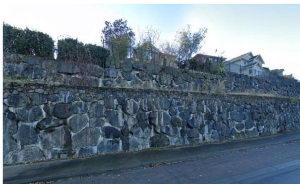
Terrace high and narrow, sidewalk between wall and parking
