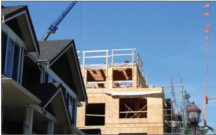
A housing development under construction on Peatt Road in Langford on May 19. (Bailey Moreton/ News Staff)
