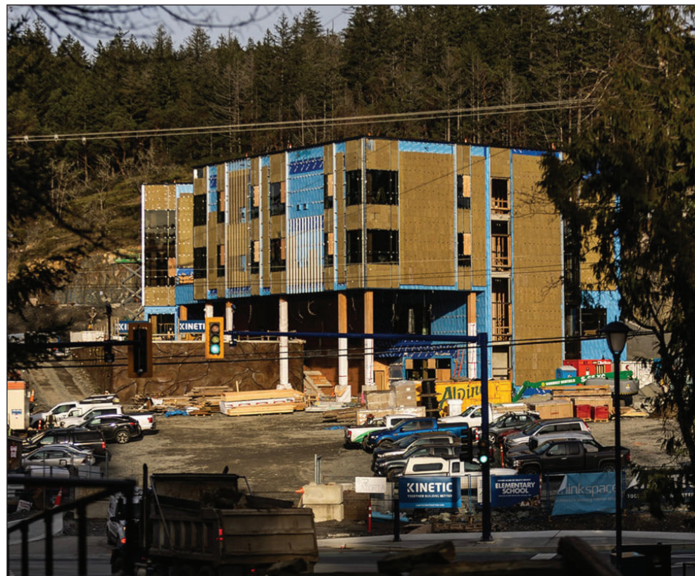
Construction continues on the new SCIANEW STELITKEL Elementary School in Langford. (Arnold Lim / Goldstream Gazette)
